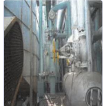
Dryer loop beside the heater battery
