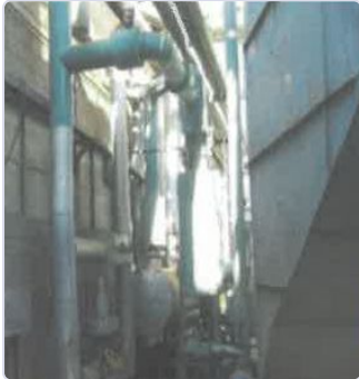
Dryer loop pipework
