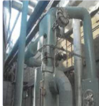
Dryer loop at the heater batteries
