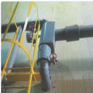
Press loop pipework
