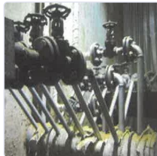
Gate valves on the condensate lines under the heat surface
